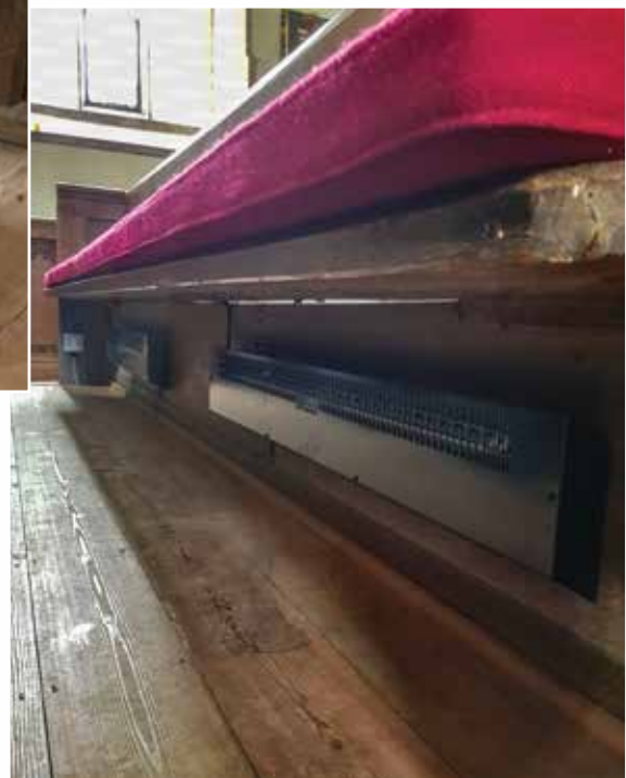
Pew heaters providing economic heating in St James Church, Egerton, Kent
