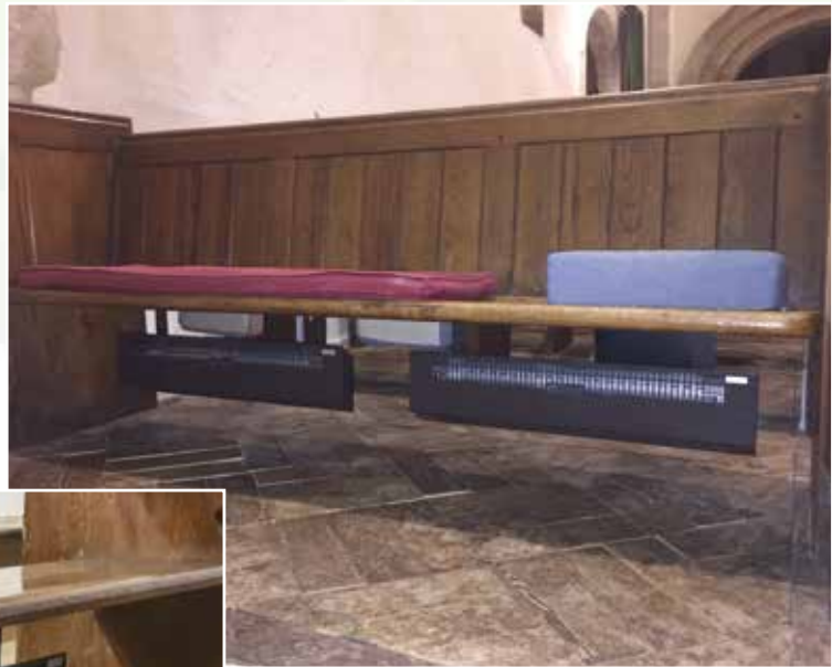
Pew heaters in a Gloucestershire church installed with suspension brackets
