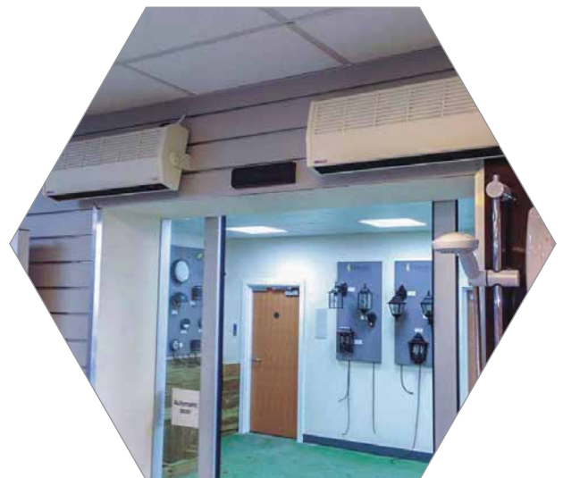
830T installed over a showroom door
