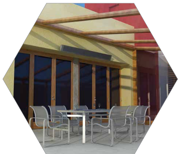
The IP44 rated ETH – suitable for permanent outdoor installation
