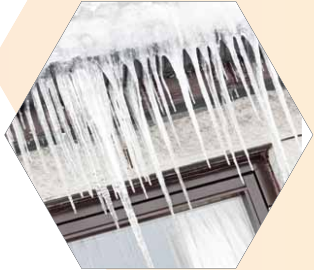
Keep gutters and downpipes ice-free
