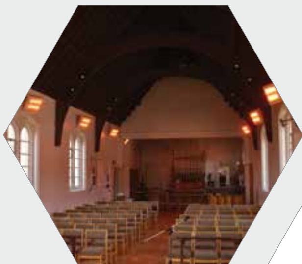
HN-3000G shortwave heaters providing instant economical heating in St Stephen's Church Barnet
