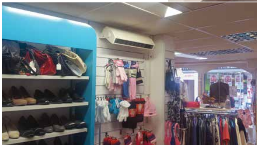
3kW heater keeping people warm in a clothing store.
