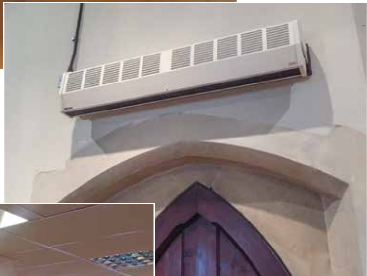
6kW heater combatting draughts in a Hampshire church
