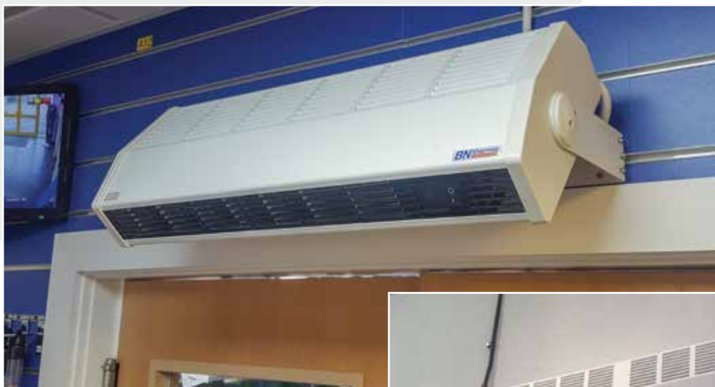
3kW heater providing a warm welcome to customers
