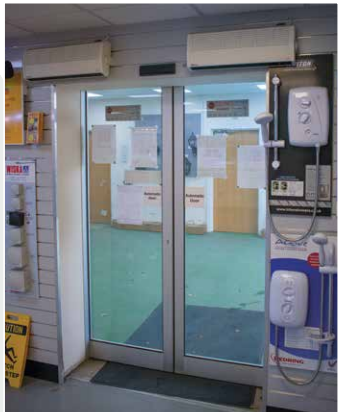
Two 3kW heaters over automatic doors
