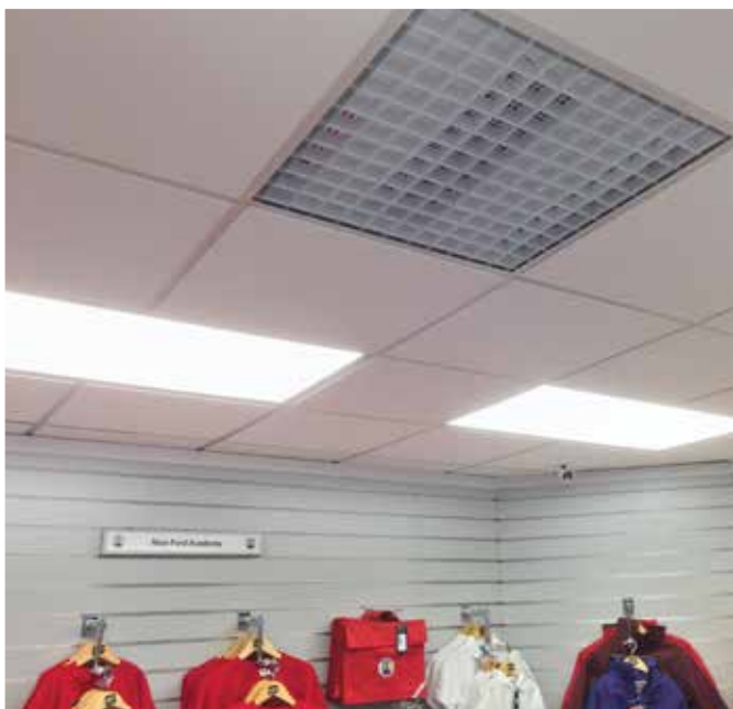
SCH heater installed in a school outfitters
