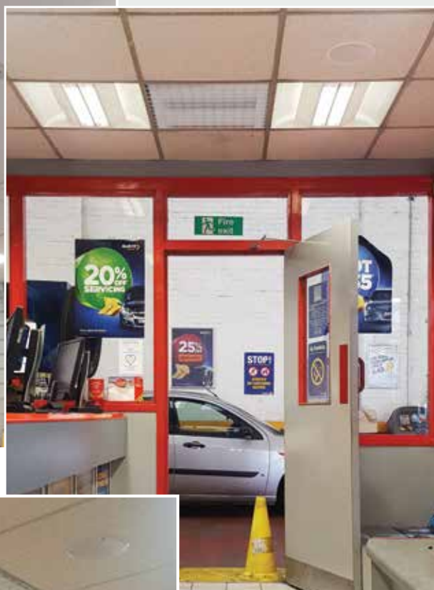
An SCH fan heater provides simple and reliable heating in a car service reception area
