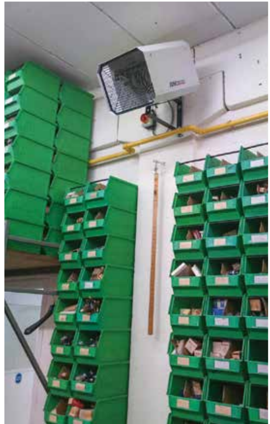
OUH2 installed in a workshop in Billingshurst, West Sussex
