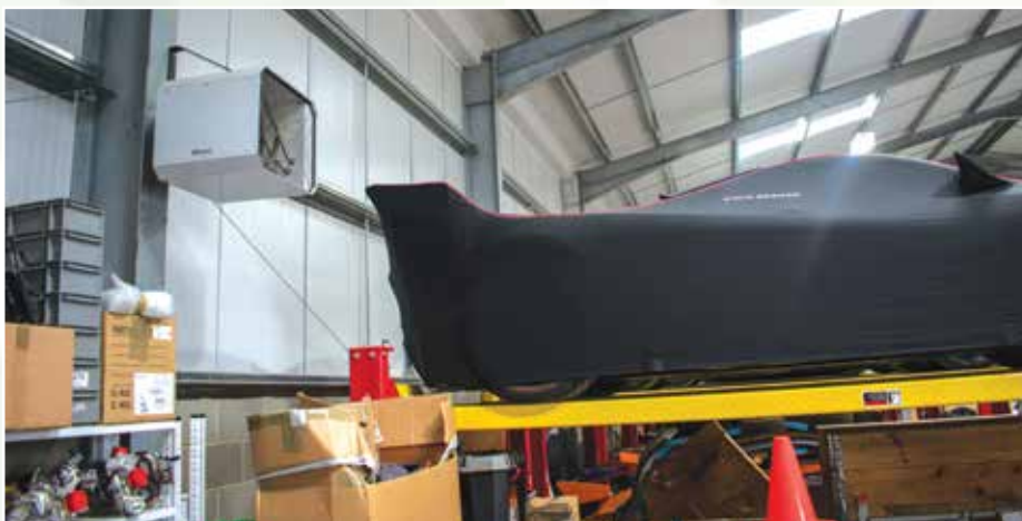
25kW OUH heaters providing frost protection in a supercar workshop
