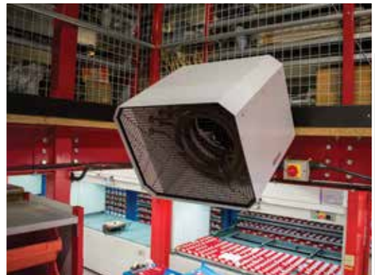
25kW industrial fan heater installed in an automotive parts store
