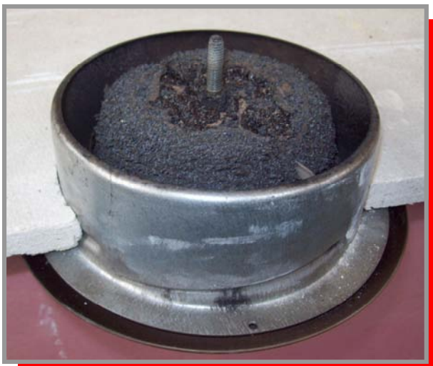
Fire Air Valve sealed after a fire
