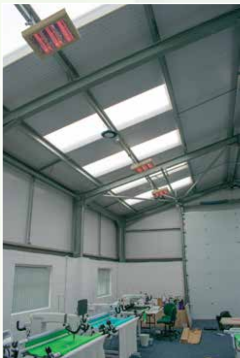
Three phase halogen heaters providing instant heat above industrial sewing machines
